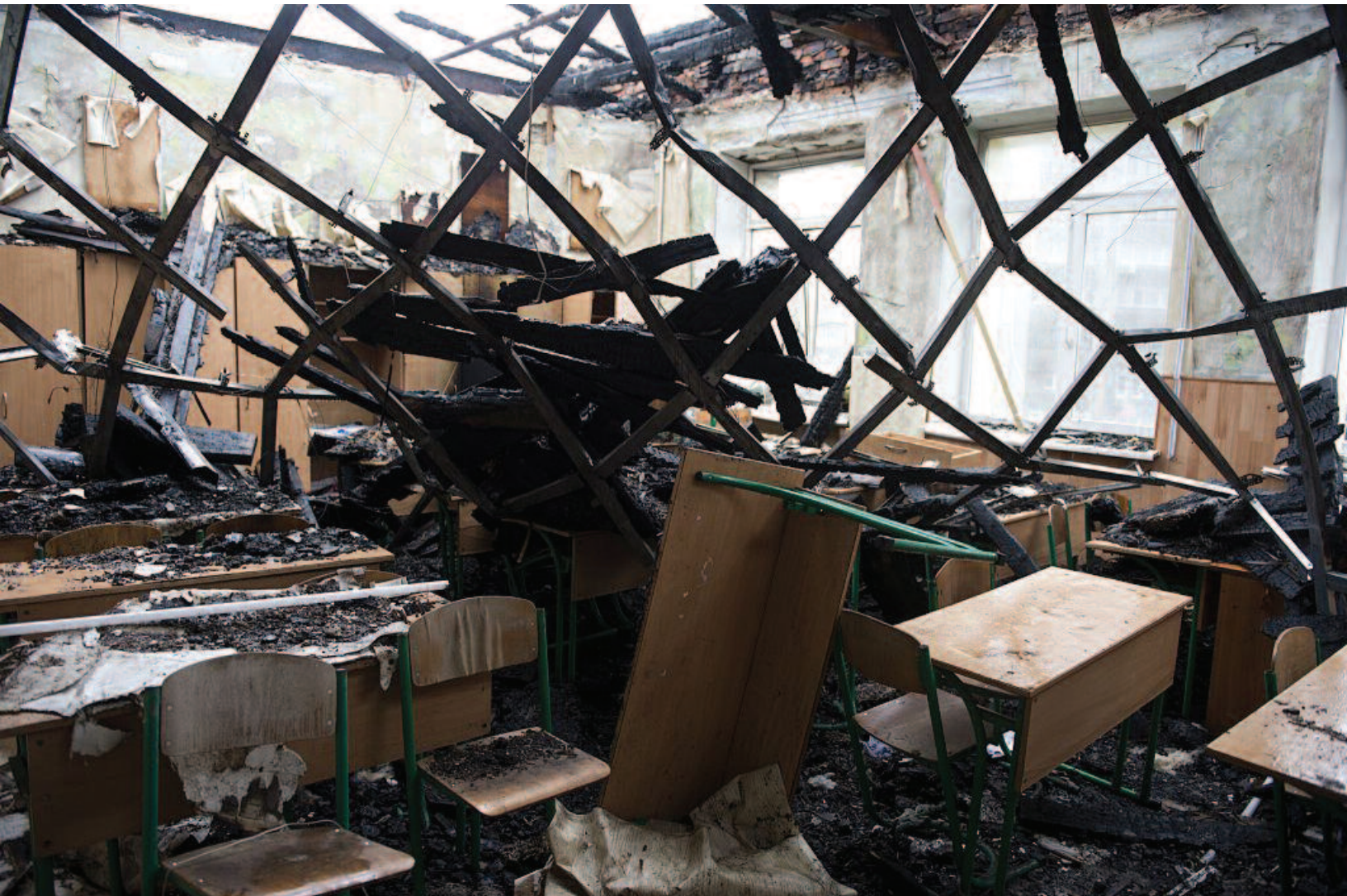
The shell-struck top floor of the Gymnasium 33 high school in Donetsk, Ukraine, hit by Ukrainian government shelling on August 27, 2014.
